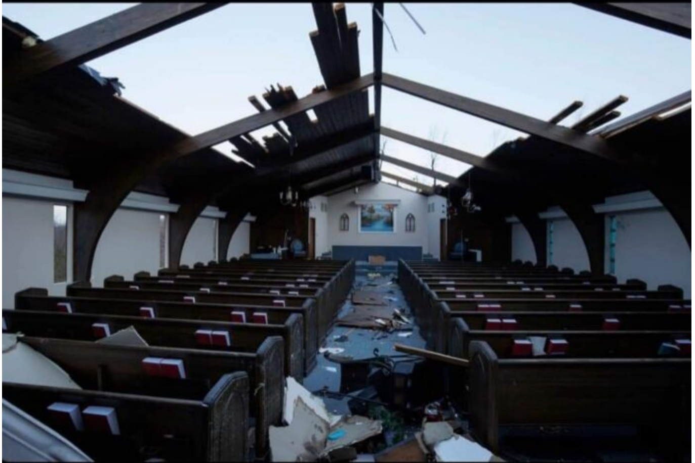
Damage to Emmanuel Baptist Church in Mayfield is seen on Saturday. Brett Carlsen/Getty Images
